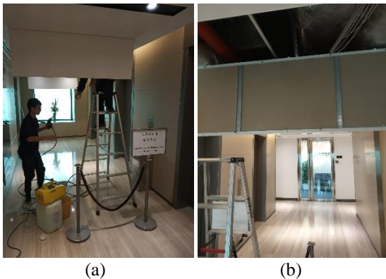
Figure 2: A routine visit to apprentices working in a commercial building (a. on-site work, b. air-conditioning facilities).
